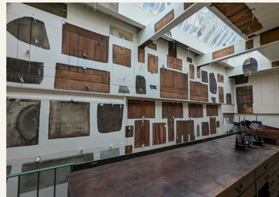
Fig.21 The south wall of the office during restoration, 2022, showing unpainted areas revealed where items were taken down that still occupied their original positions. © Sir John Soane's Museum, London. Photo: Matt Tidby.
